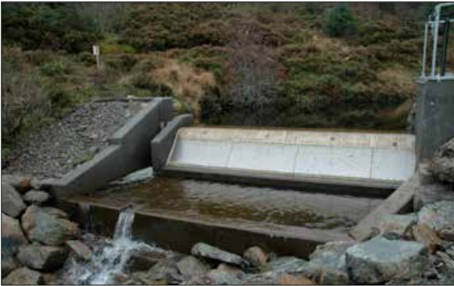
The intake, with the screen to filter the water and the outlet on the left hand side to allow the compensation flow.
