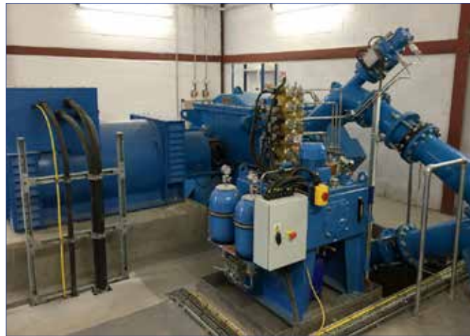
Inside the turbine house - the turbine, the generator and in the third photo, the control panels.
