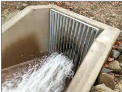
The out-take, where the water leaving the turbine house is returned to the stream.
